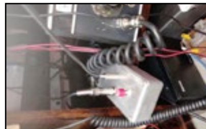
This is the junction box with a PTT switch. The coiled cable connects the junction box to the TR-7.
